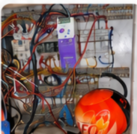
CONTROL SYSTEM MAINTENANCE
