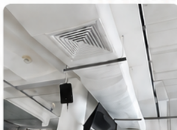
AC DUCT SYSTEM
