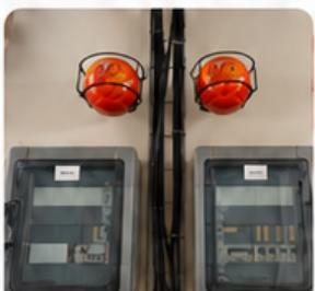
ELECTRICAL PANEL SERVICING
